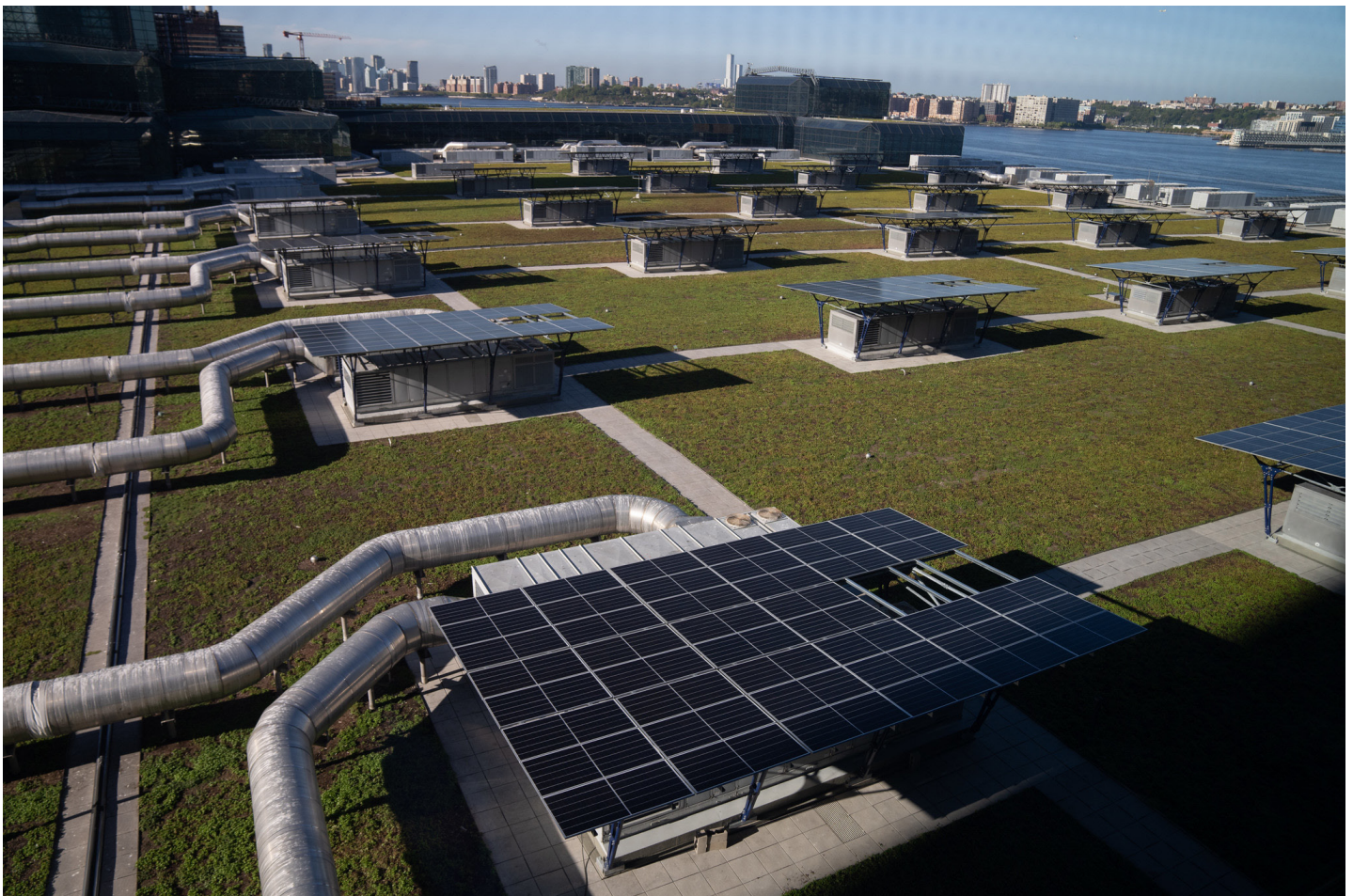
Solar panels, Javits Center, New York City, NY.
